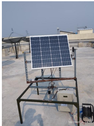
Figure 2. Solar Tracking System Dual Axis
