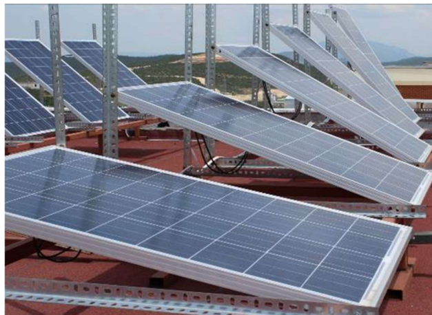
Figure 2. Fixed PV panels [14]
