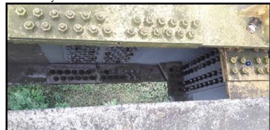
Figure 7. Rusty bolt on tied rod
