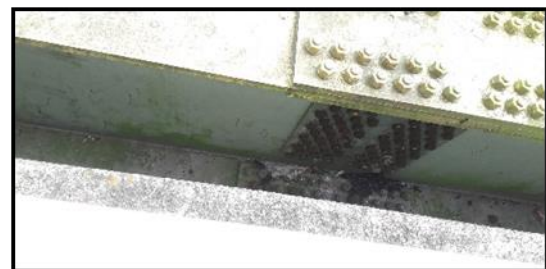
Figure 8. Rusty bolt on tied rod
