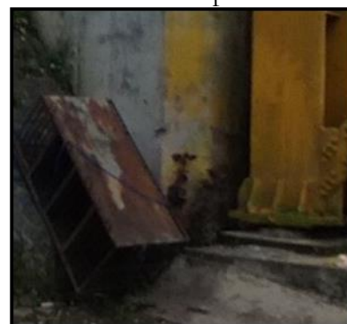
Figure 9. Photo fractional abutment
