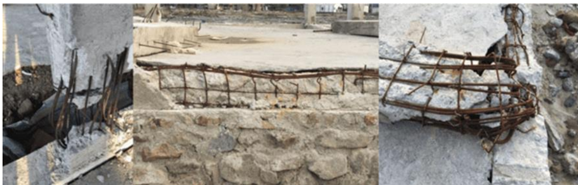
Figure 1. Failure in shear reinforcement installation on reinforced concrete beams and columns (S. P. Tampubolon et al., 2022)
