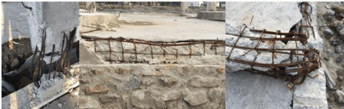
Figure 1. Failure in shear reinforcement installation on reinforced concrete beams and columns (S. P. Tampubolon et al., 2022)
