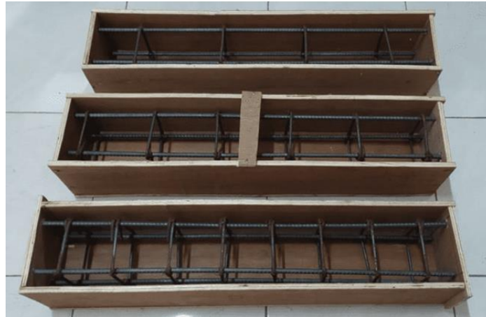
Figure 7. The assembled specimens of reinforced concrete beams with formwork are ready for casting
