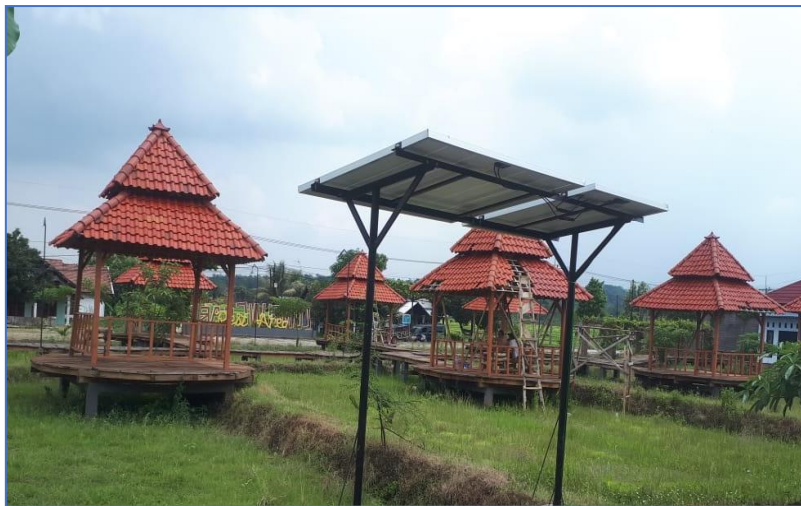
Gambar 14 Panel Surya terpasang
